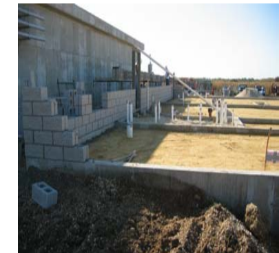
Process Equip Building
