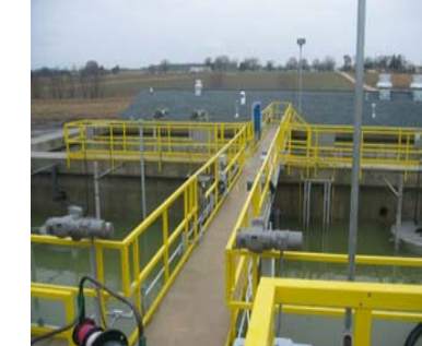
Tanks Ready for Service
