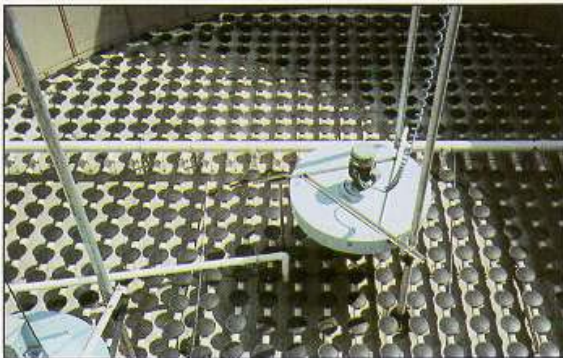
Typical SBR (Batch) Aeration System, three cycles per day
