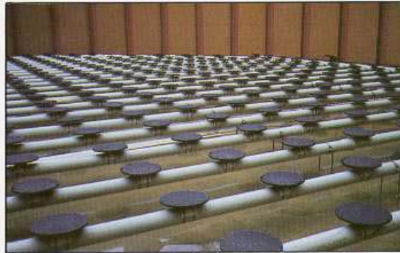
Large continuous aeration system
